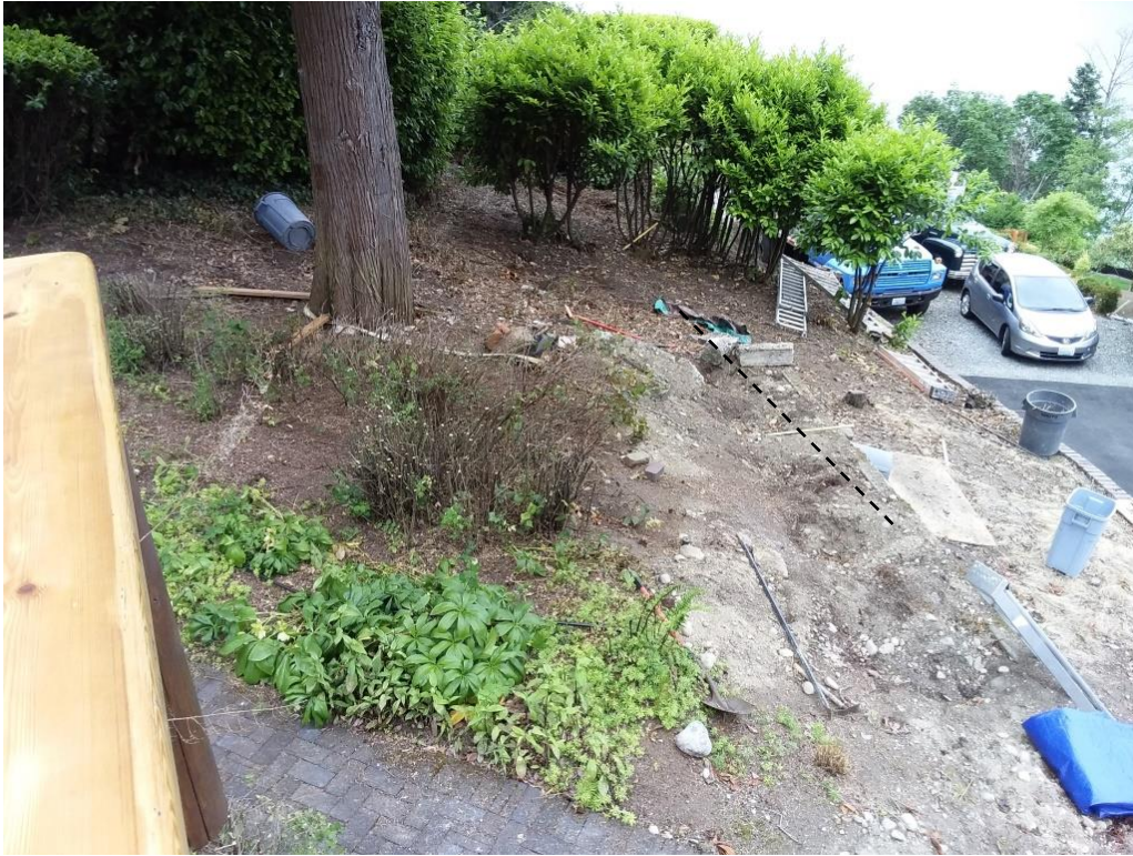
Figure 10. Photo showing the location of the retaining wall on the west side of the #13 cedar (black dashed line).
